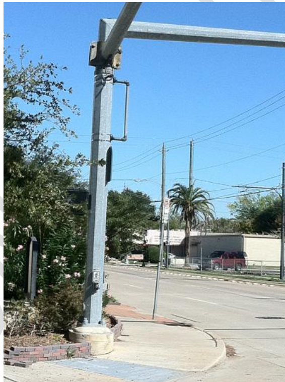
Figure 4: Pole Mounted Equipment, San Jacinto @ Wichita
